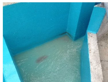
ARMOURGUARD PW in a waste water treatment plant at a chocolate factory
